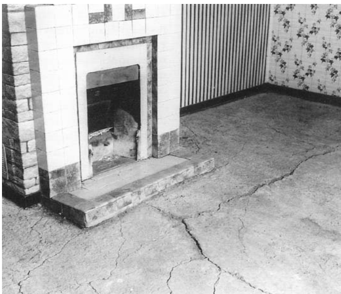
Figure 1: Distortion and cracking of a concrete floor slab caused by sulfate attack. Damage is greatest in front of the fireplace where water, carrying sulfates from underlying hardcore, has been drawn through the slab by heat from the fire.
