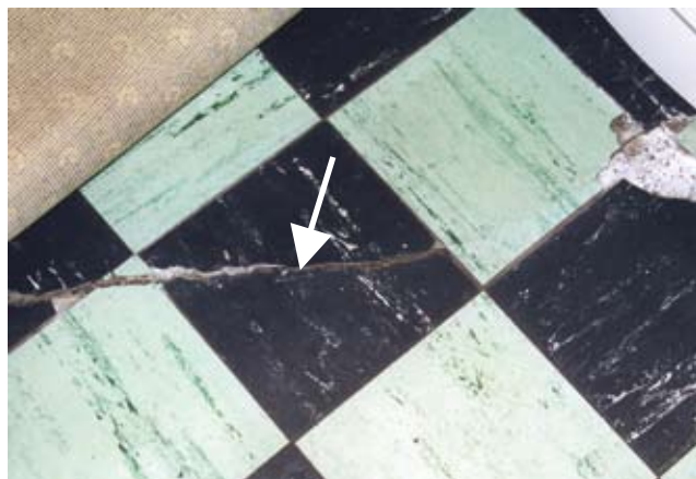
Figure 9: Stepped crack in floor of 1950s house that may indicate sulfate attack. The unevenness could be felt through the (rolled back) carpet.
