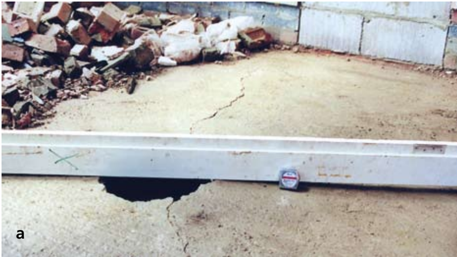
Figures 7(a, b & c): Sulfate-attacked oversite concrete that was laid over plaster contaminated brick rubble beneath a suspended wooden floor (here removed together with the sleeper walls). (a) An improvised straight edge shows some 50 mm doming of the oversite concrete that lifted brick sleeper walls and wooden floors.
