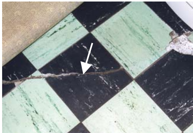
Figure 9: Stepped crack in floor of 1950s house that may indicate sulfate attack. The unevenness could be felt through the (rolled back) carpet.
